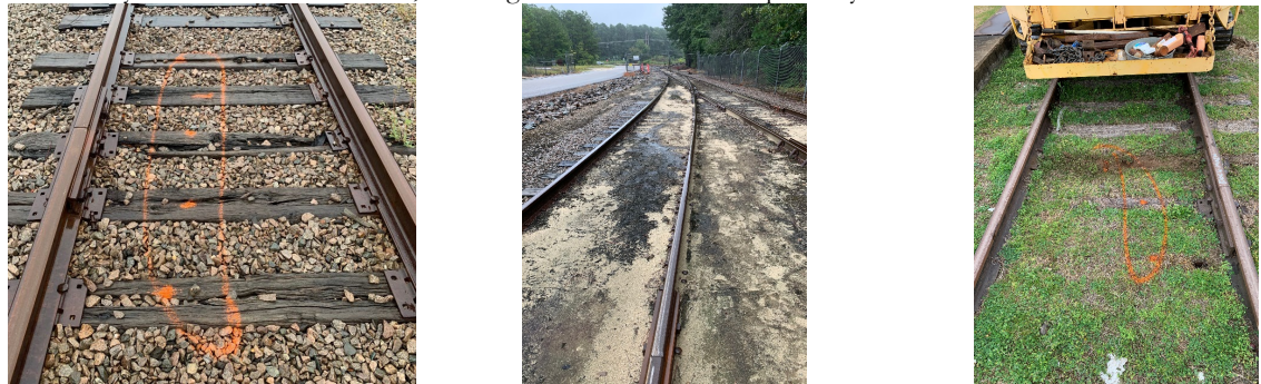
a) Joint and defective crossties in a row. b) Poor drainage and fouled ballast. c) Fouled ballast. Figure 4. Examples of common defects found by the ERDC Railroad Track Evaluation Team on Army Track.
